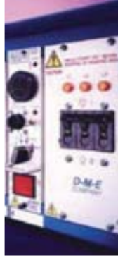
TAS shown in Communications Mainframe
